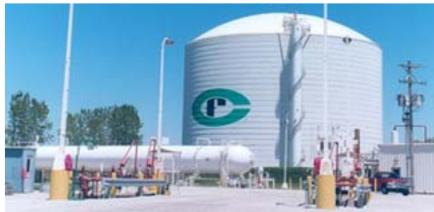
Figure 7. “Atmospheric” refrigerated liquid anhydrous ammonia (NH 3 ) tank stores 190,000 MWh as 30,000 Mt of NH 3 fuel. Total capital cost ~$15M; ~ $0.10 / kWh
